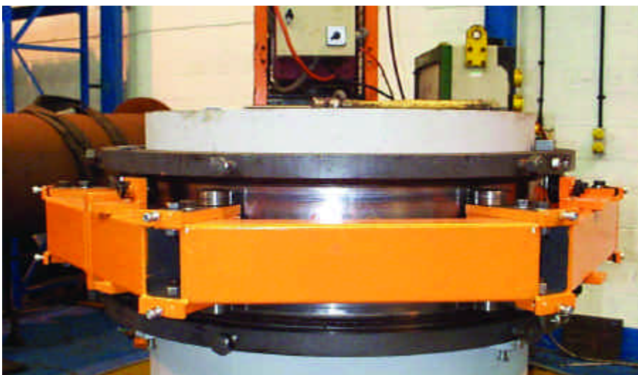
A split-bearing sleeve, shown above, was designed by First Hydro Company and contractor Furmanite to help guide a milling machine as it rotated around the main turbine shafts during a bearing replacement project at the 1,728-MW Dinorwig Pumped-Storage Power Station.
