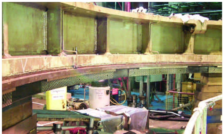
This photograph shows a new self-lubricating Lubron AQ30 regulating ring bearing in place at the Dinorwig power station in the United Kingdom, the last step in First Hydro Company's goal to create a completely grease-free turbine.
