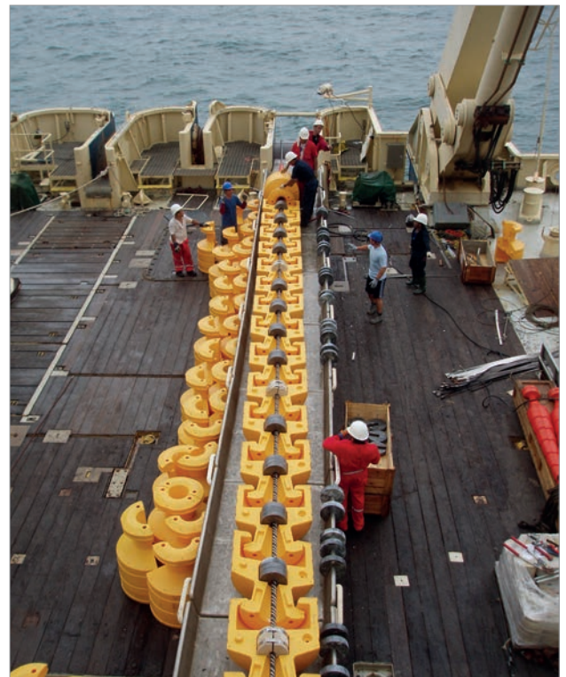
Polyspace installation on offshore vessel
