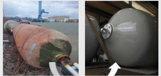
Successful refurbishment of a foam fender, restored to near-new condition: Ideal form of recycling.
