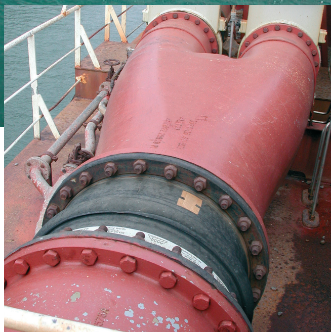
Expansion joint in loading line ▶
