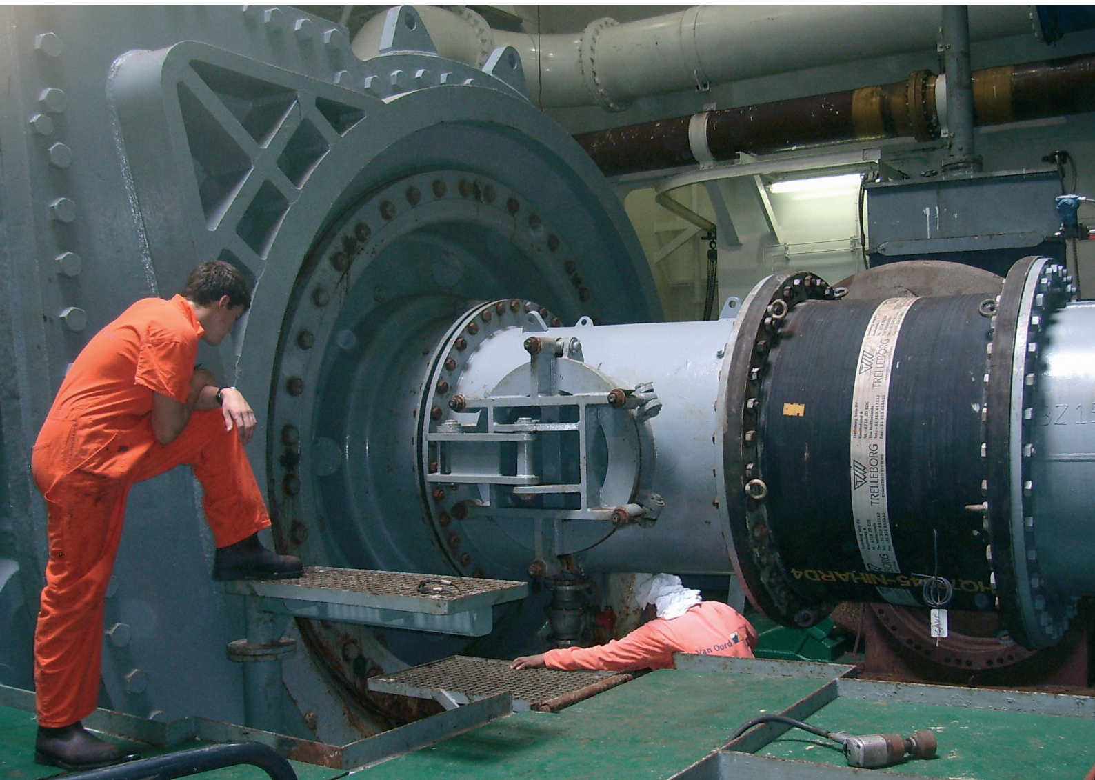
▲ RockTrail® expansion joint in pumphouse Replaces a pair of slipflanges Cures leakage in pumphouse and reduces wear on impeller and piping
