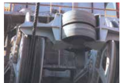
In this configuration, no maintenance of any kind has been necessary since installation.
