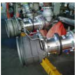
Oil and gas flow control
