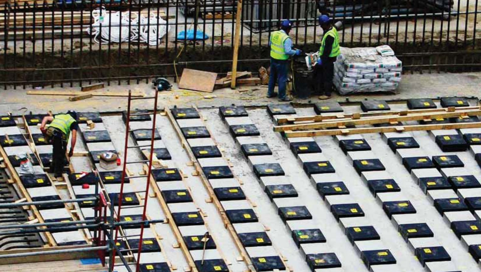
Park House rests on 363 rubber bearings installed at the sub-basement level, under the building's two central cores.
