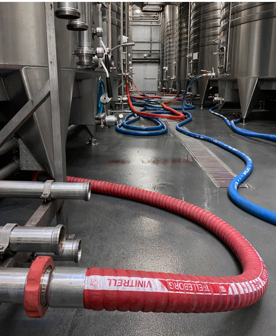
Left: Hoses used for transfer in wineries.
