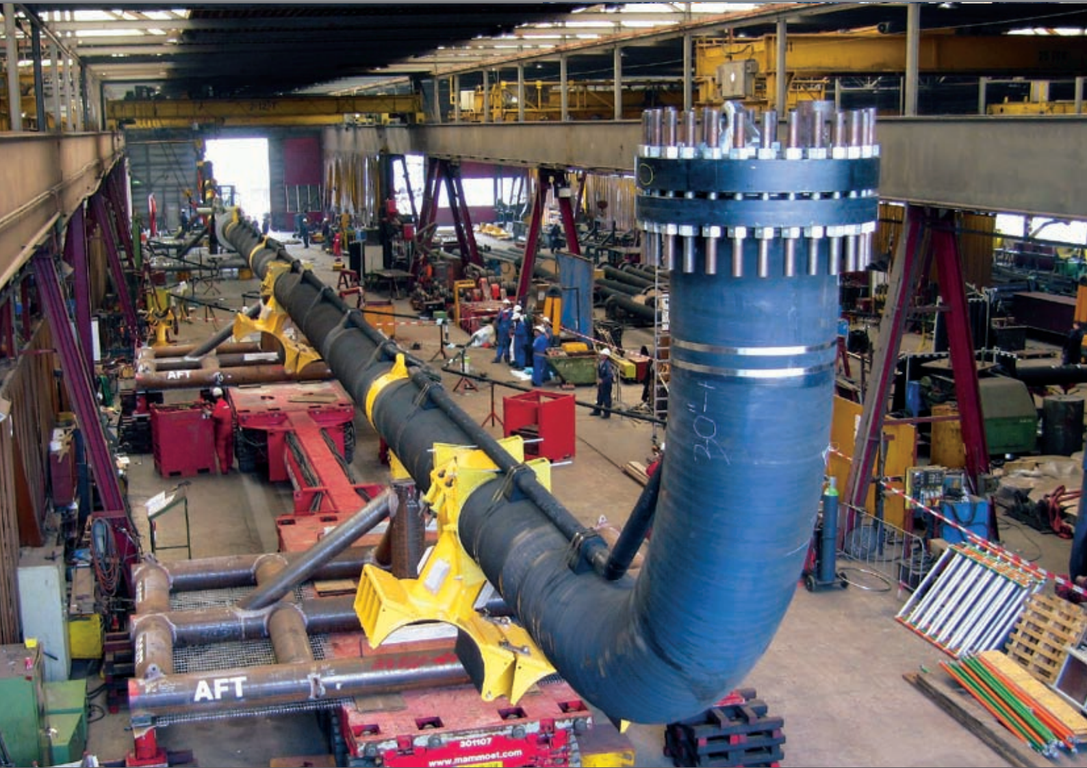
Riser of Leman 'A' platform, Shell UK. Source Fabricom.
