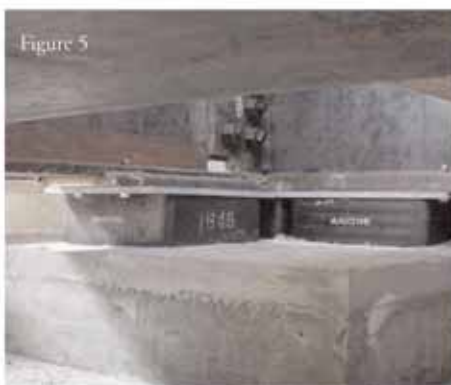
Andre Resilient Natural Rubber Bearings installed under The Disney Concert Hall, Los Angeles.
